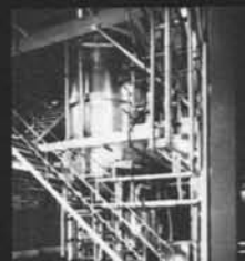
Rosedowns Semi Continuous Deodoriser processing cocoa butter at a rate of 4,000 lbs/hr.
